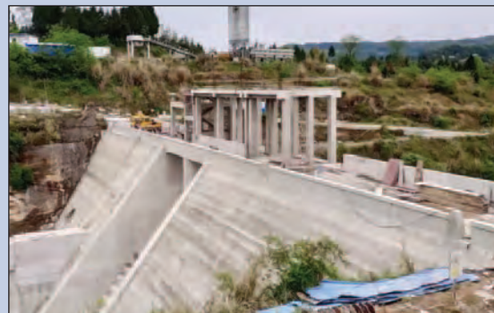
Jinjigou dam, under construction in China, one of several examples of a cemented material dam, presented by Dr Jia Jinsheng. He spoke about the characteristics of CMDs, including safety against overtopping, and the possibility to be built on non-rock foundations.
